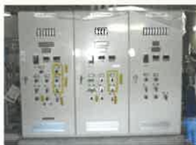
各種盤(制御盤) Various panels (control panels)
