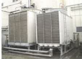
業務用空調設備 Industrial air-conditioning equipment
